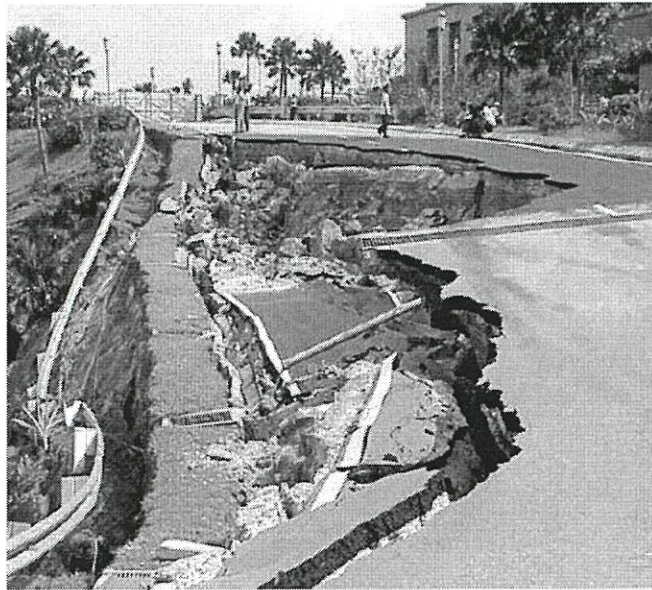
(a) The top portion of the failed slope
